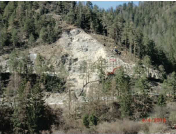
Figure 13 View of the unstable slopes along Serfauserstrasse.
