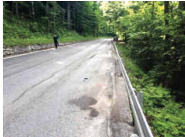
Figure 2 Photo of the state road DC3 (section 015) at km 2+060 before remediation works. Tension cracks at the crown of the landslide Dedin are visible on the asphalt.
