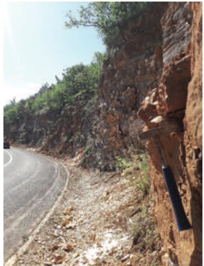
Figure 2 Example of the slope with a high degree of undercutting (segment from km 18+950 to km 19+150)
