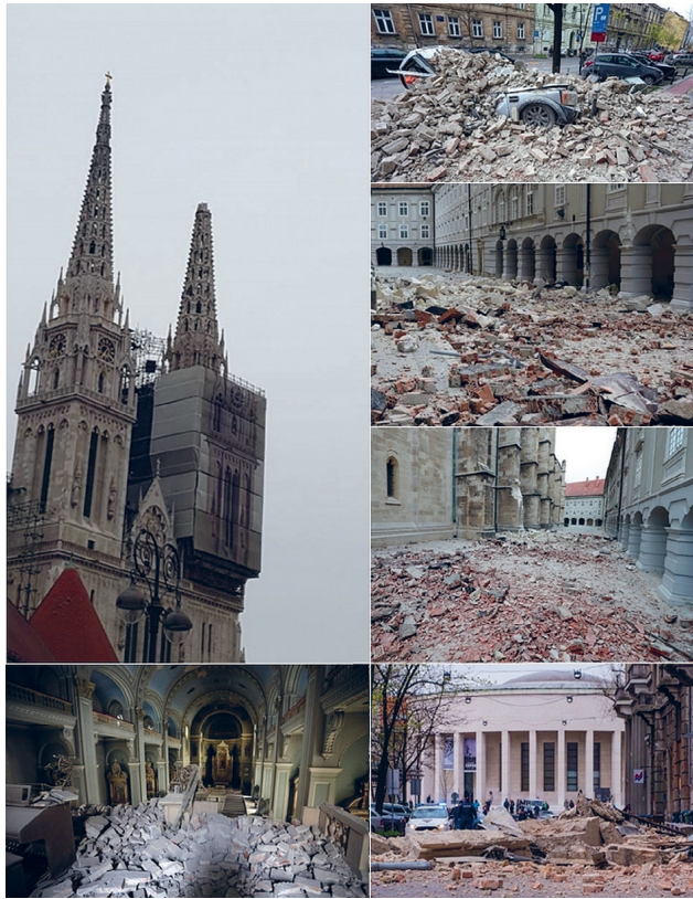
Figure 1. Photos of damage in Zagreb caused by the 22 March 2020 earthquake (from Markušić et al., 2020).
