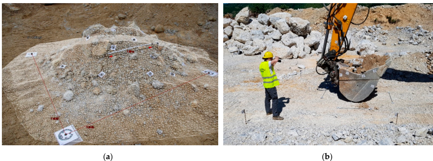
Figure 2. (a) Measuring volume of the bucket load and (b) angle of repose of material.
