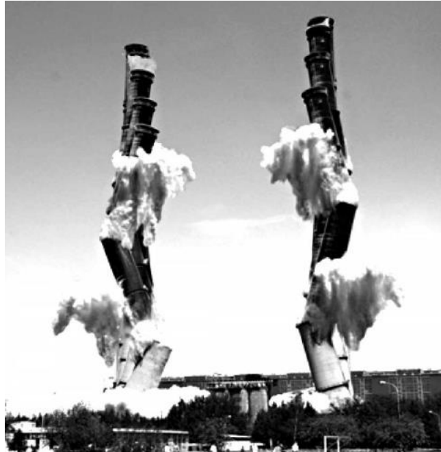
Slika 5-4 Cik-cak kolaps dimnjaka 1 i 2 ((Melzer,2015 )
