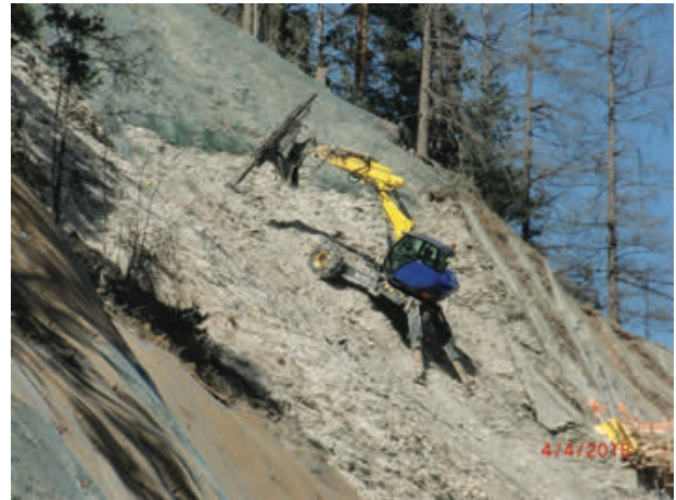
Figure 10 A walking excavator in action, drilling the next row of anchors, while being already protected from the top, as the high-tensile steel mesh is already installed.
