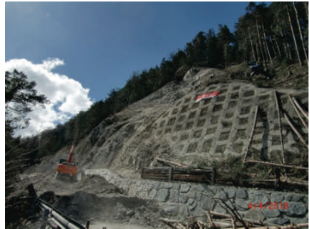
Figure 8 View of the beginning of works to clear the road from the landslide mass.
