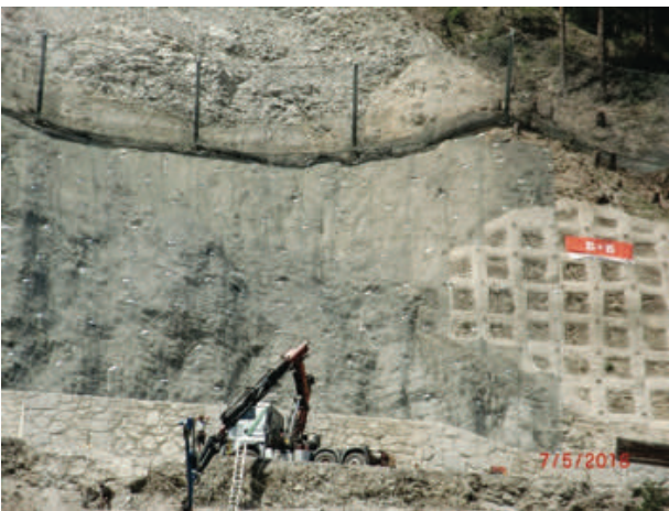
Figure 14 Drilling truck starting on the stabilisation works at the bottom part of the Serfauserstrasse instability.
