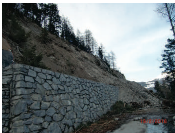
Figure 4 View from the blocked Ladiserstrasse, where a large part of the slope failed after the extreme weather conditions in January 2018.
