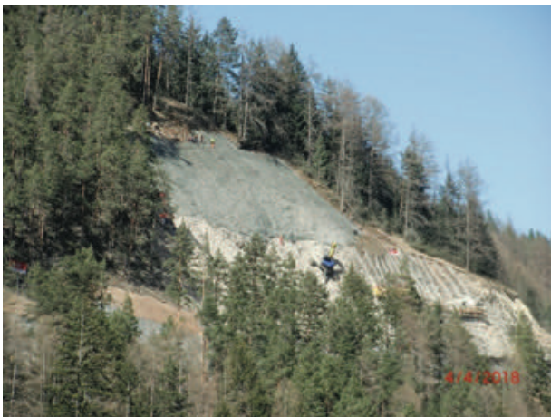
Figure 9 View of the unstable slope at Ladiserstrasse, where the first part of anchoring and mesh deployment is completed, allowing secure works underneath to be completed.
