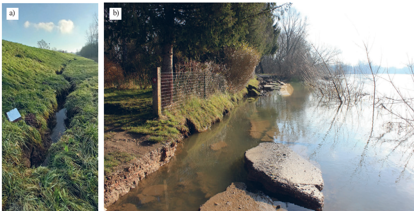
Figure 6. Lateral spreading and associated processes: a) failure of the flood embankment in Sisak (observation point Si-03); b) road failure in Letovanić (observation point RMT-35).
