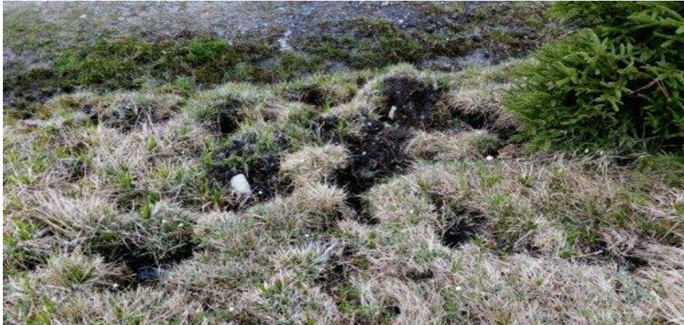
Figure 6-4 Field photo showing cracks near the end of profile p2
