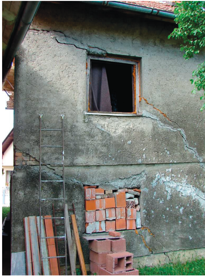
Figure 5. Damage caused by sliding (photo by D. Tibljaš).
