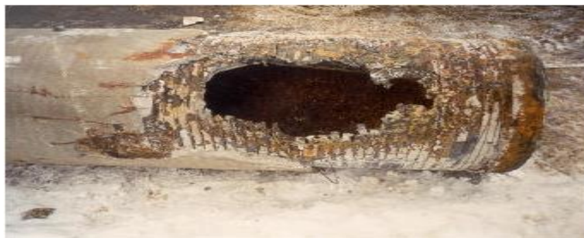
Slika 3-5. Korozije cjevovoda u tlu ( https://corrosion-doctors.org/SoilCorrosion/ , 14.08.2020.).
