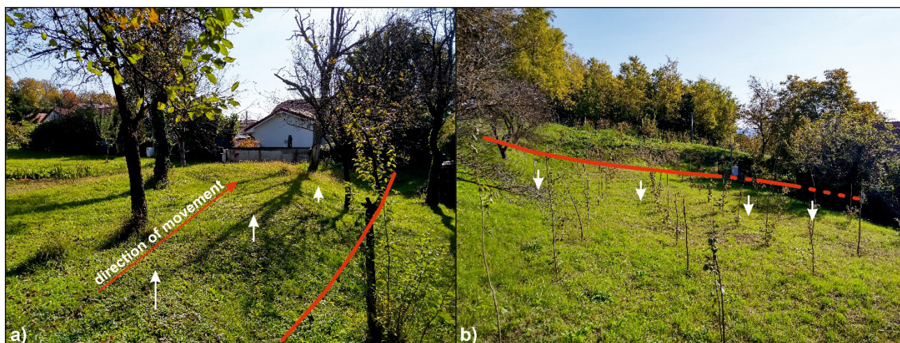
Figure 8: Vertical deformations at the Kostanjek landslide: a) uplift of the material (white arrows) at the western boundary (red line); b) subsidence (white arrows) along the minor scarp (red line) in the eastern part of the landslide
