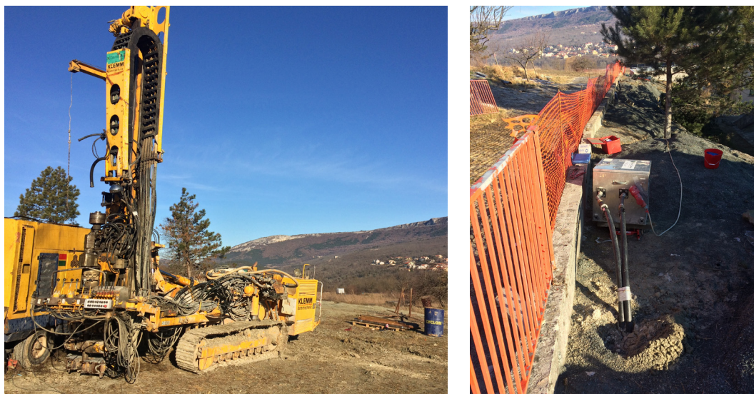
Figure 3: left) Experimental test site – drilling operations; right) Thermal response test equipment during testing
