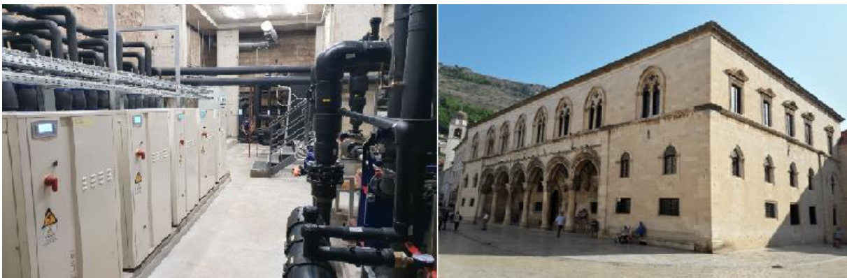
Slika 3-9. Sustav dizalice topline u Dubrovniku (Seadrion Project, 2018b)
