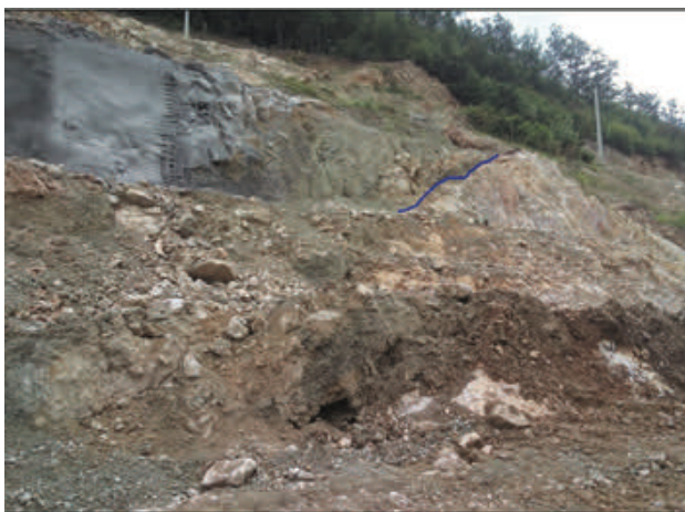
Figure 4 Left boundary of an active landslide.
