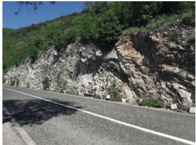
Figure 1 Example of the slope with major launching features present (segment from km 19+300 to km 19+490)
