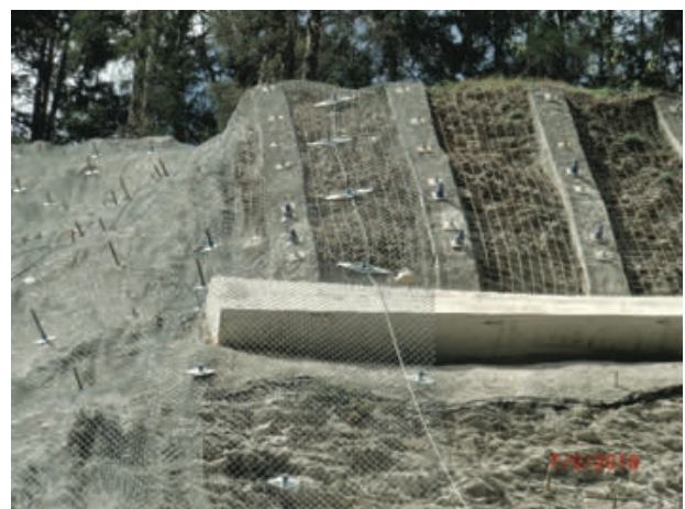
Figure 12 Stabilisation of the concrete ribs that were undamaged during the slope failure, with a concrete anchor beam and high-tensile steel mesh cover. Note the larger spike plates, belonging to the TECCO system, which can support higher loads.
