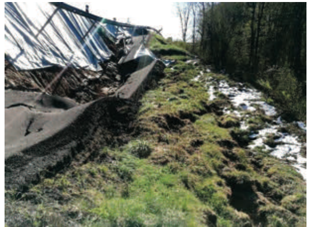
Figure 4 Main scarp of the Dubravci landslide.
