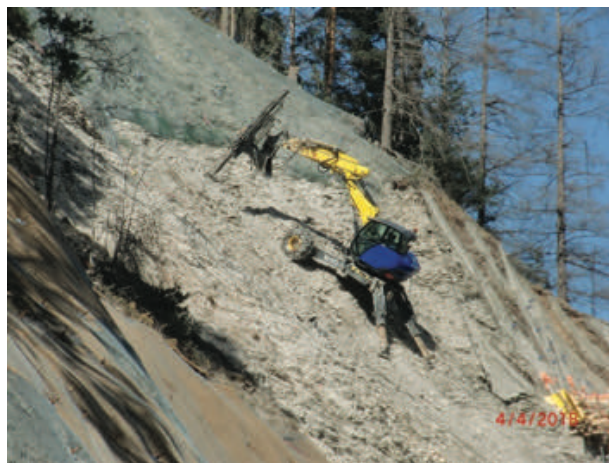
Figure 10 A walking excavator in action, drilling the next row of anchors, while being already protected from the top, as the high-tensile steel mesh is already installed.
