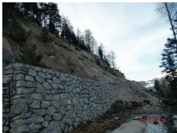
Figure 4 View from the blocked Ladiserstrasse, where a large part of the slope failed after the extreme weather conditions in January 2018.
