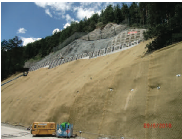
Figure 15 Final works underway at the Serfauserstrasse, with a highlight on the greening mat along the bottom part of the road.
