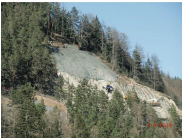
Figure 9 View of the unstable slope at Ladiserstrasse, where the first part of anchoring and mesh deployment is completed, allowing secure works underneath to be completed.
