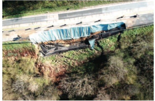
Figure 3 Aerial view of Dubravci landslide on the state road DC3 (section 015) at km 2+060.
