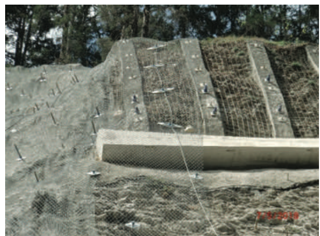
Figure 12 Stabilisation of the concrete ribs that were undamaged during the slope failure, with a concrete anchor beam and high-tensile steel mesh cover. Note the larger spike plates in this section, belonging to the TECCO system, which can support higher loads.
