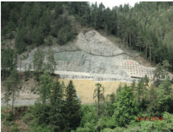
Figure 20 Serfauserstrasse stabilised slope, with a rockfall barrier at the top, anchored high-tensile steel mesh in the middle and greening mats in the bottom part of the slope.
