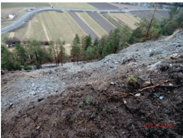
Figure 7 View from top of the landslide along the Serfauserstrasse, approximately one month after the event.
