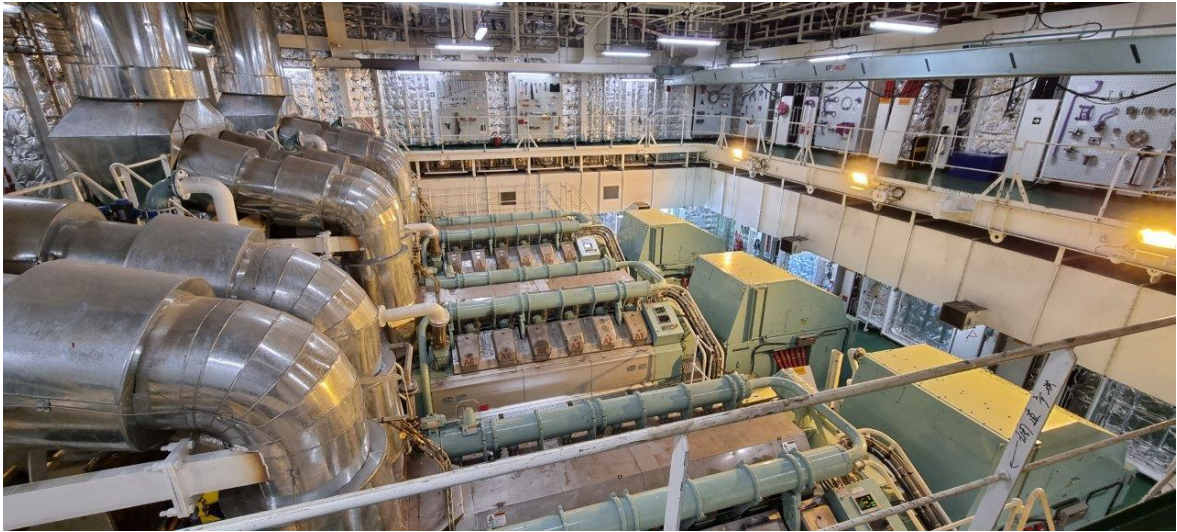
Figure 1-5 The three Wärtsilä 12V34DF gensets in the engine room of the LNG terminal, side view (LNG Hrvatska, 2024)
