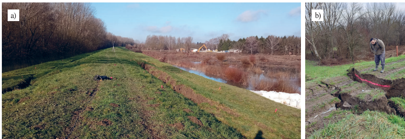
Figure 7. Subsidence and lateral spreading of the embankments near the Sava river: a) in Sisak (observation point Si-03); b) in Palanjek (observation point NP-21).
