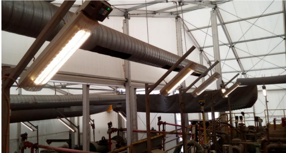
Slika 3-20. Instalirana rasvjeta EATON 92 LED 400 (Crosco, 2017b)
